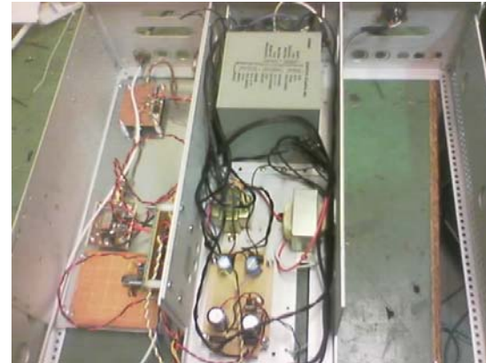
Rack unit: TX modules and power supply
